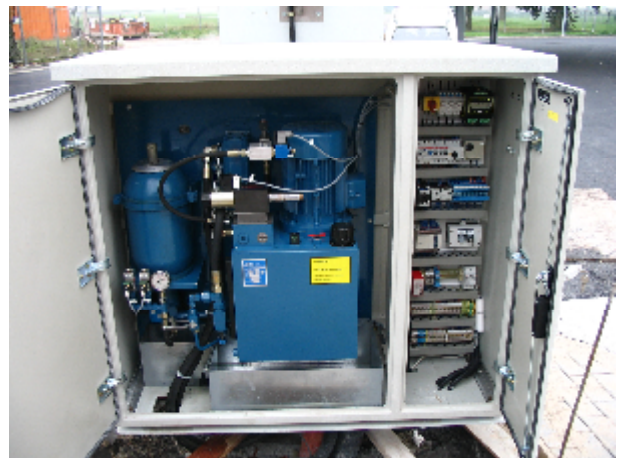
Reference Control unit
